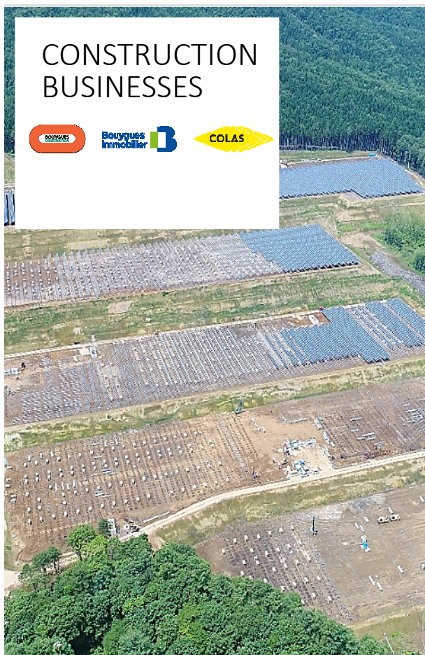
13.7 MW solar farm in Noheji, Japan
